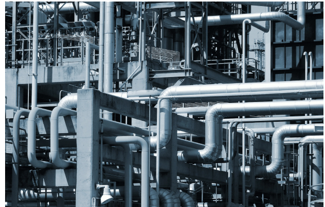
Refineries are a typical application where fire and gas detection systems are found
