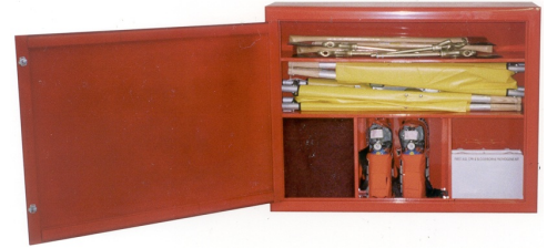
Emergency Equipment Cabinet w/ First Aid Supplies
